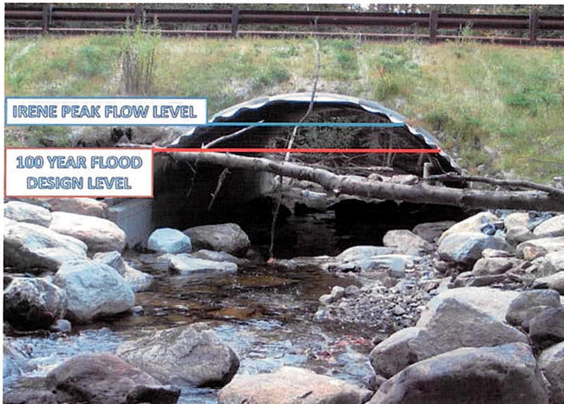
Figure 5. Stream simulation design culvert at Jenny Coolidge Brook, installed in June 2010, showing height of 100-year design discharge in red and height of Tropical Storm Irene flood level in blue. Photo credit: Brian Austin, Green Mountain National Forest.
