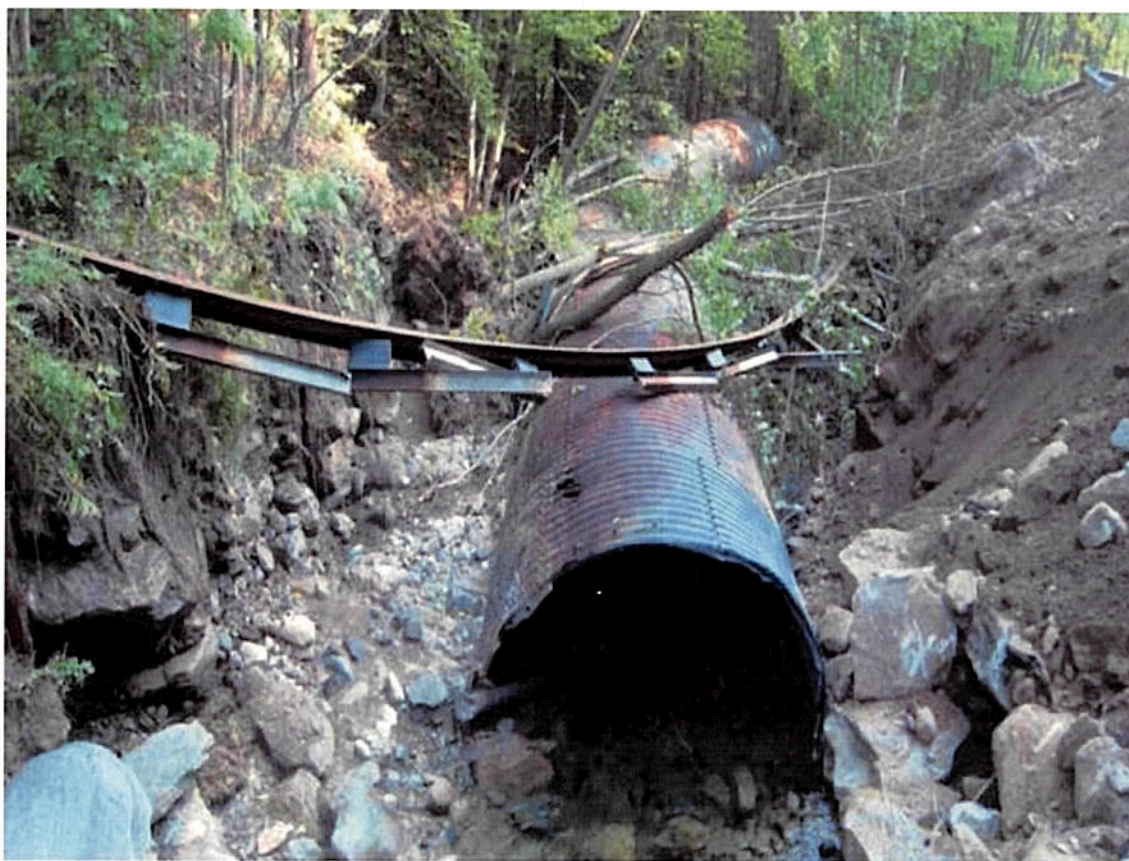
Figure 1. Road failure at a 3-m culvert placed within a 6-m bankfull width stream, Green Mountain National Forest. Photo credit: Dan McKinley, Green Mountain National Forest.
