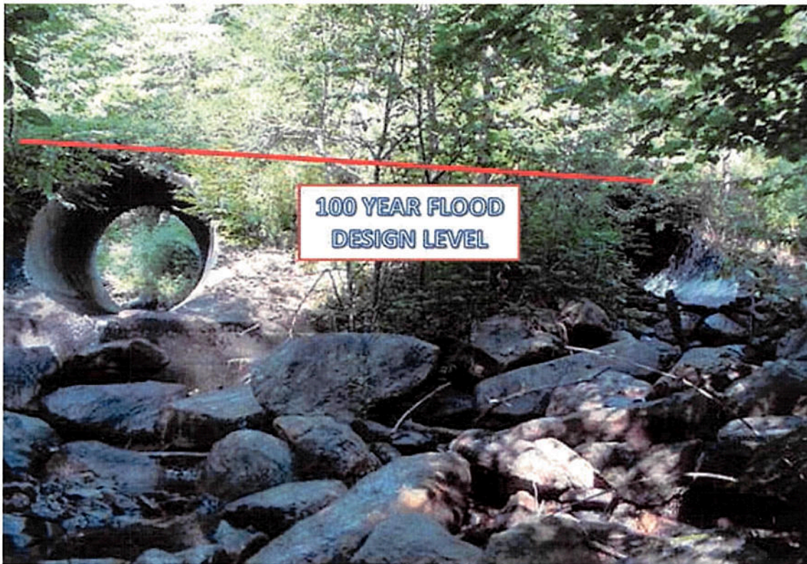
Figure 4. Typical hydraulic design double culvert over Jenny Coolidge Brook, May 2010. Green Mountain National Forest showing estimated height of 100-flood design discharge in red. Photo credit: Brian Austin, Green Mountain National Forest.
