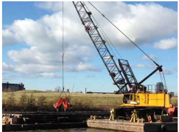
Dredging and capping contaminated sediments in the City Ship Canal, which connects to the Buffalo River, helped restore crucial aquatic habitat for fish, birds and other wildlife.
