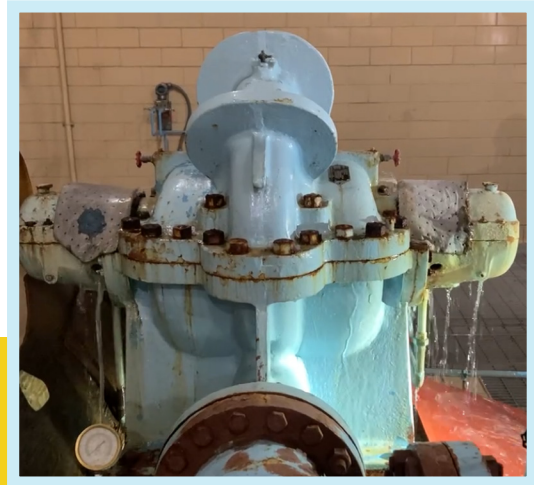
Photo 1: Corroding and leaking pump valve in Troy.
